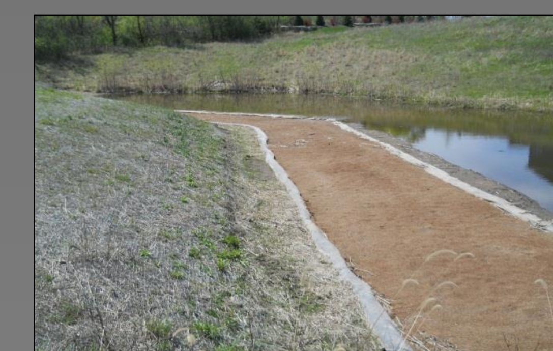
Figure 12. An iron enhanced sand filter is shown between the water and grass
